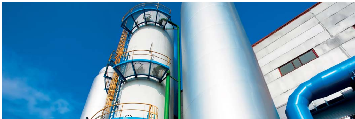
Air Separation Plant
